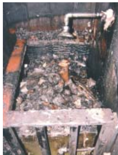
Close-up of sauna heater
