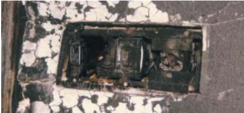
Switch plate: From left to right are the heater switch, the on/off light, the interior sauna light and the temperature control.
